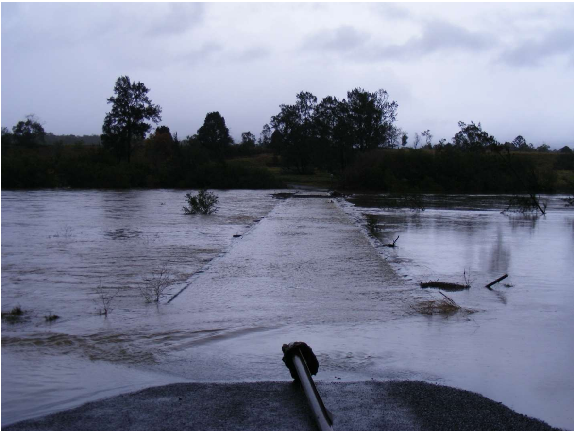
Photo 7: Flooding of Turners Flat Bridge (Time and date unknown, 2011 event)
